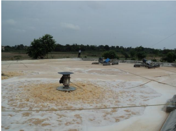
Aeration Tank (Biological Reactor)
