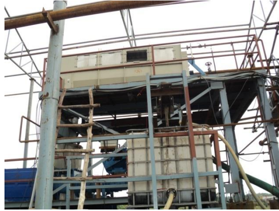
Sludge thickener and decanter
