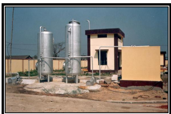
Effluent Treatment Plant
