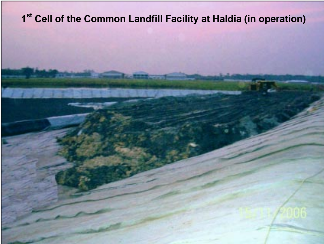
First Cell of the Common Landfill facility at Haldia (in operation)
