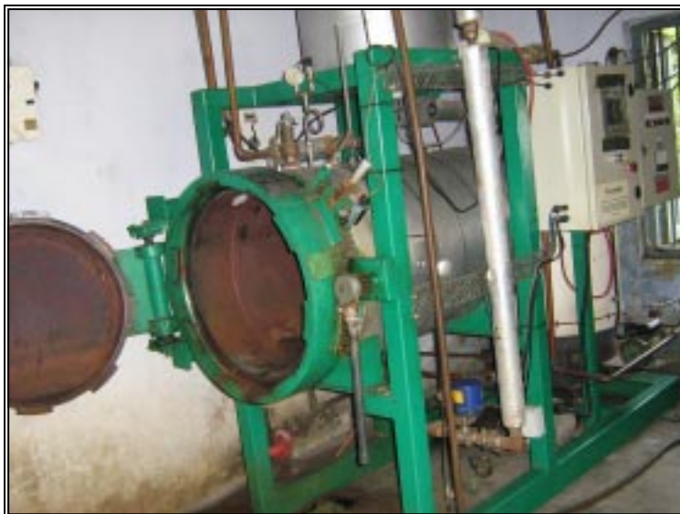
Autoclave installed at JNM Hospital-Kalyani under WBHSDP, Health Department, Government of West Bengal for treatment of non-anatomical bio-medical waste
