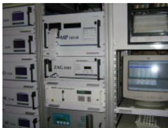
Inside of Automatic Air Quality Monitoring Mobile Van
