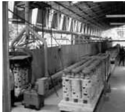
Oil Fired Tunnel Kiln
