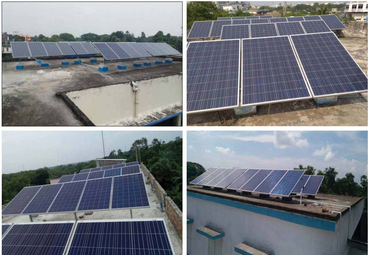
Figure 24.8: Rooftop Photovoltaic Cells Installed by WBPCB
