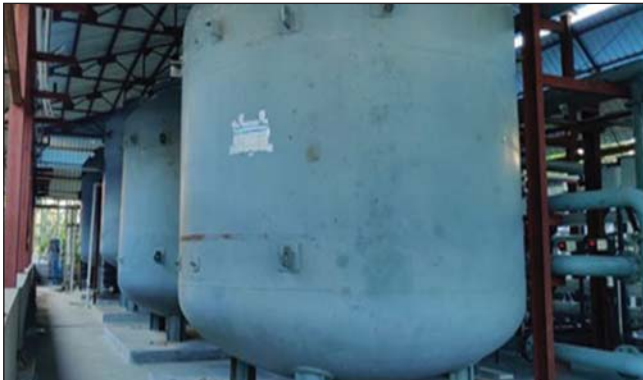
Filtration and Softener Units
