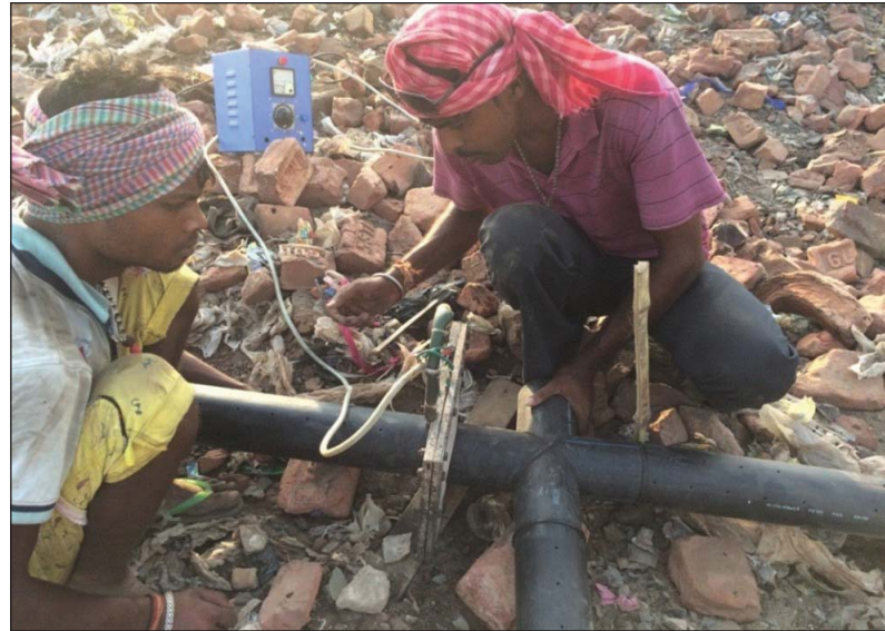
Figure 24.22: Laying and Jointing of HDPE Pipes of Different Diameters for Gas Collection and Transport
