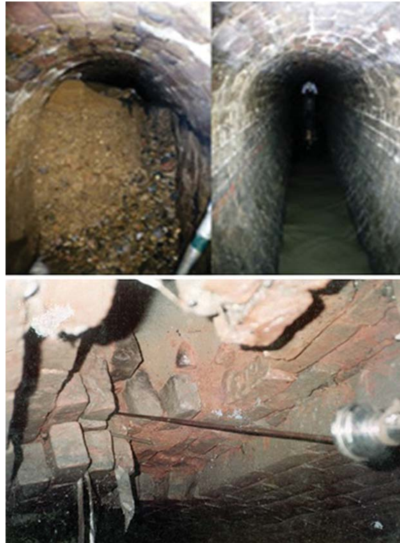
Figure 19.15: The accumulation of silt inside underground sewer channels (left image) and the cleaned sewer channel (right image). The bottom image shows the bricks dislodging off the sewer channel wall.
