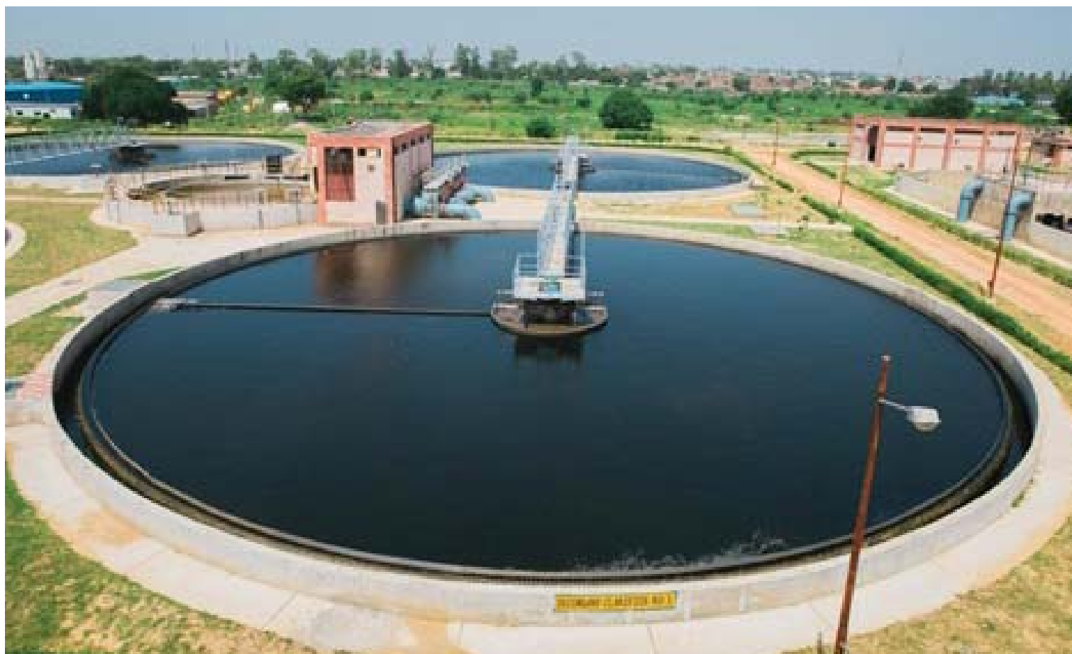
Figure 19.10: Wastewater Treatment at Nilothi in West Delhi with a Capacity of 90,000 M 3 per day
