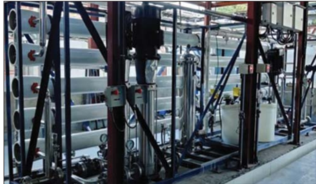
Reverse Osmosis Plant
