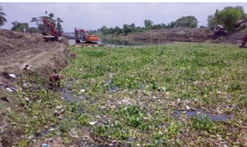
Figure 19.17: The Sewer Canals of the City of Kolkata, Clogged by Outgrowths and Solid Wastes
