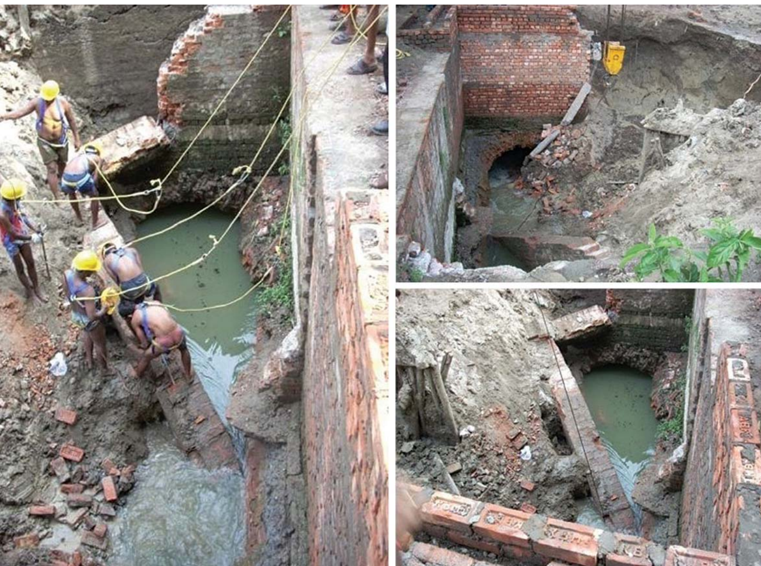
Figure 19.16: Complete Underground Brick Sewer Collapse and Damaged Drainage System in Kolkata
