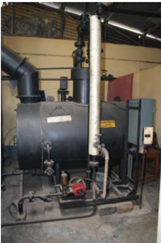
New oil-fired boiler
