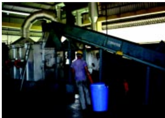
Incinerator of the Common Biomedical Waste Treatment and Disposal Facility at Howrah
