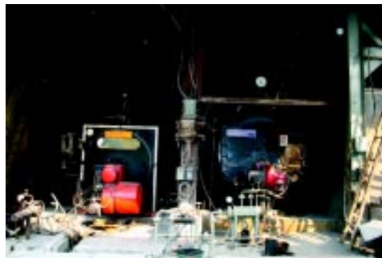
New oil-fired boiler
