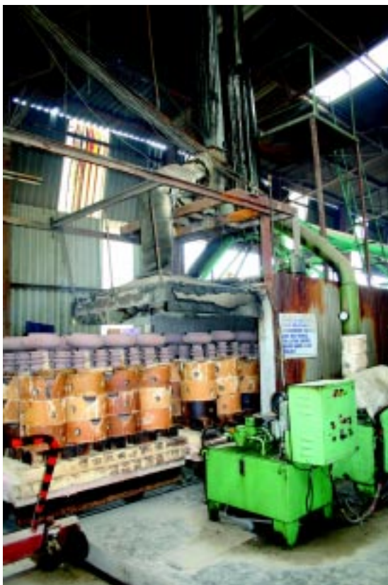
New oil-fired tunnel kiln
